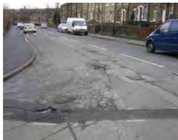
Potholes, image courtesy of David Mazurke
