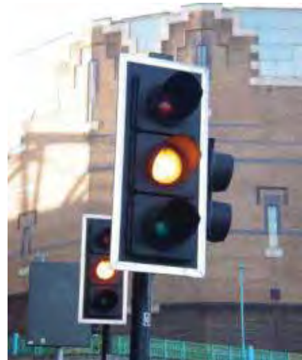
Traffic signals, image courtesy of Atkins
