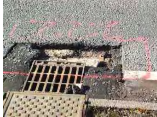
Damage to ironworks, image courtesy of Atkins
